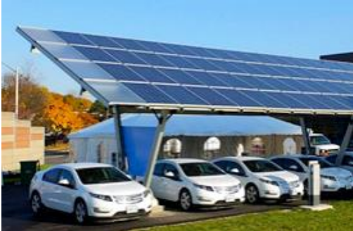
Charging site integration (chargers, solar and energy storage)
